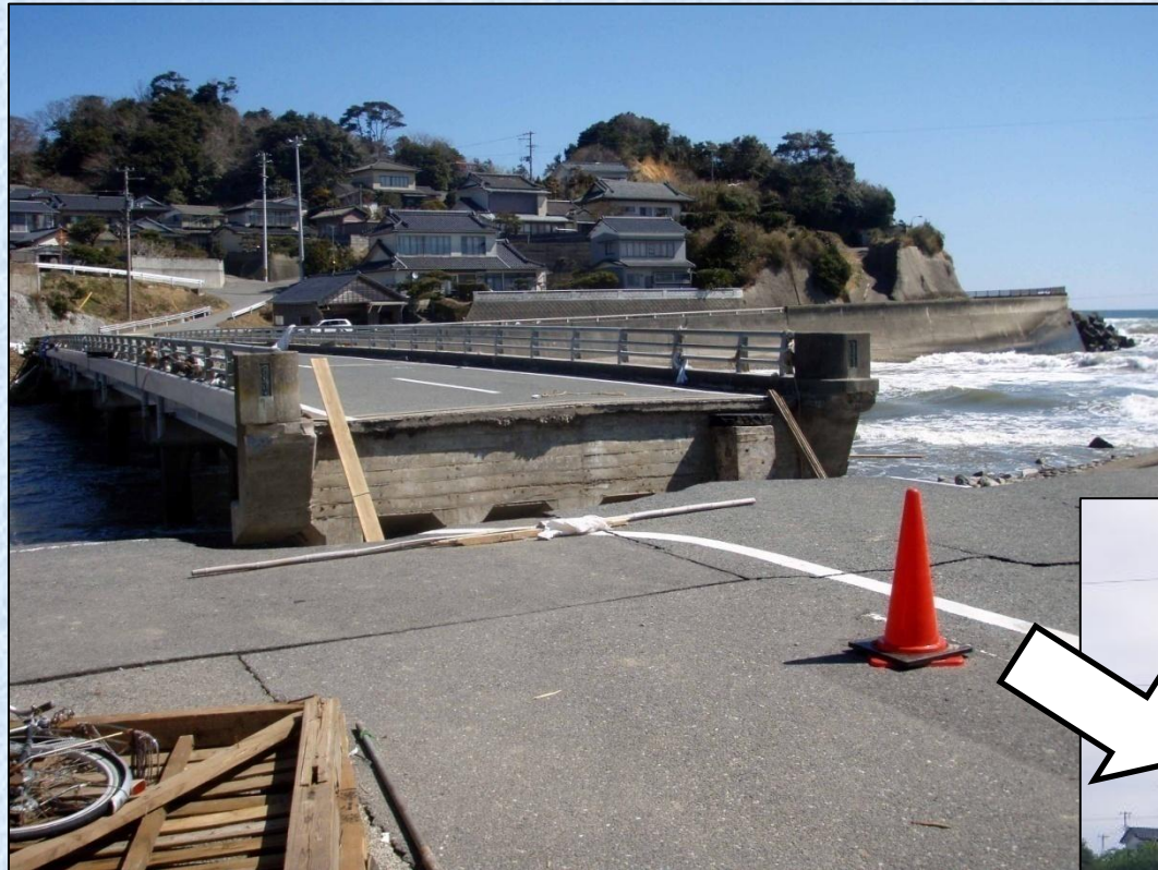
Bridge Abutment Collapses, Hisanoma Prefectural Road
