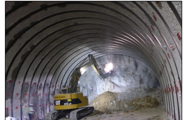
The Sekiba Tunnel in the Kawamata Town section on the National Road Route 114 was opened on 2 Mar. 2022
