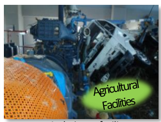
A drainage facility in Soma city
