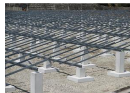
Support frames for mega solar generators
